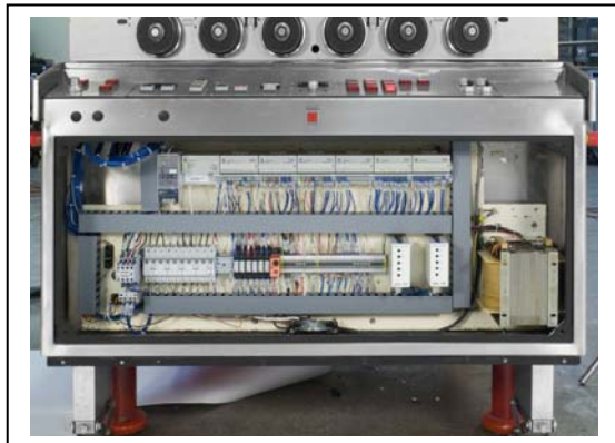
New MKIV Front Control Cabinet
